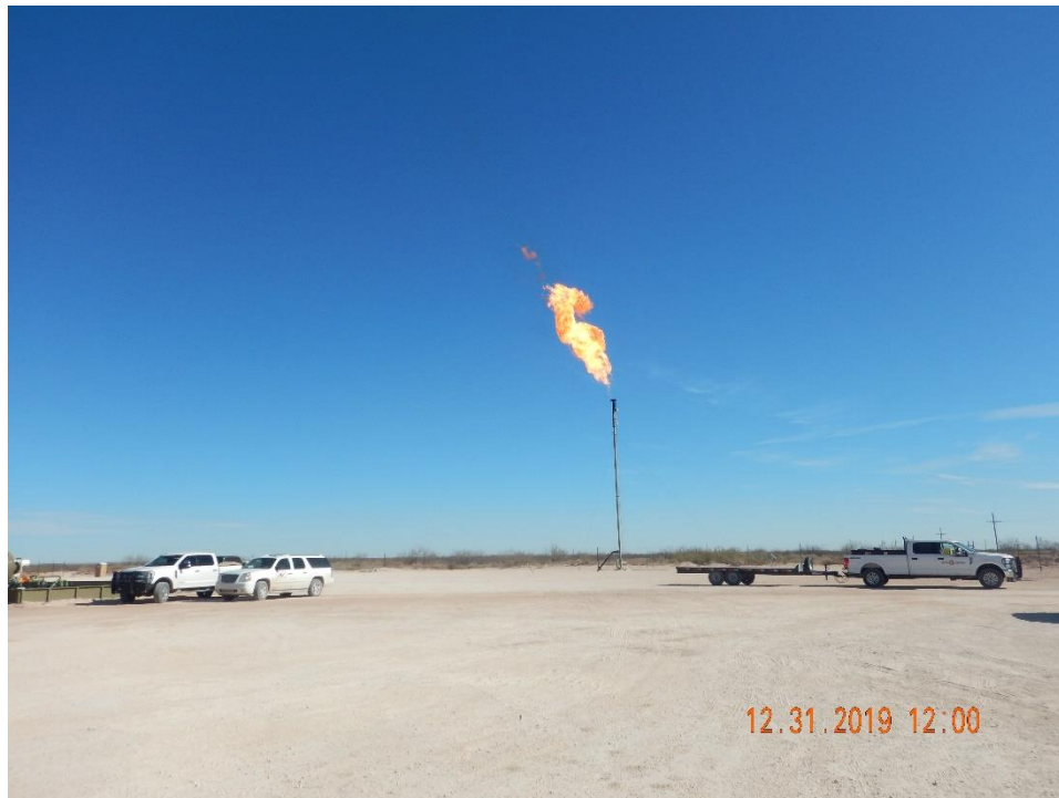
An unauthorized flare at Ameredev’s Nandina facility, photo by AQB inspectors taken on Dec. 31, 2019.
